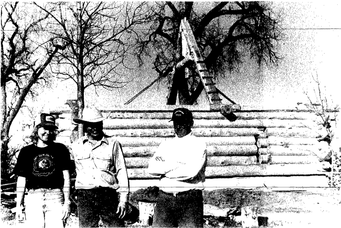
Nancy Lunzer and Brian Nelson are in the process of building their dream home east of Wayne. Log home builder and craftsman Jim Christensen, right, has several projects of this type to his credit. The logs for the home were taken from Nancy's family's farm in Minnesota and were shipped to Wayne county for final assembly.
